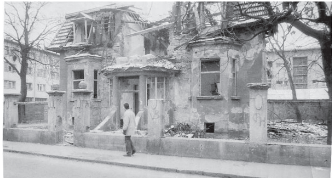
Figure 2.28. A photograph of Villa Božić in the 1980's, showing traces of time and neglect that gradually led to its demolition
